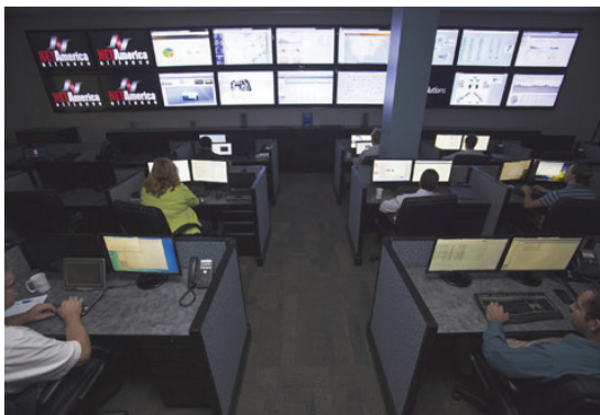
An inside peak at CHR’s Network Operations Center (NOC) in Houston.
